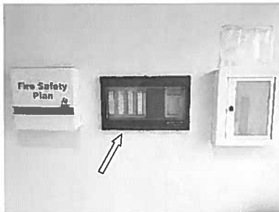
View of the "Notifier" remote annunciator panel.
