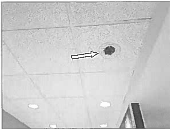
View of the water staining and black staining (i.e., potential mould growth) in the ceiling tile noted in the washroom of the Site Building.
