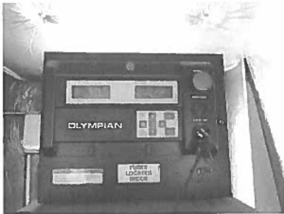
View of the "Olympian" natural gas-fired emergency generator.
