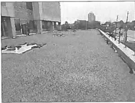
General view of the future green roof system overtop the PVC single-ply membrane roof system noted on the lower roof area atop the south portion of the Site Building.
