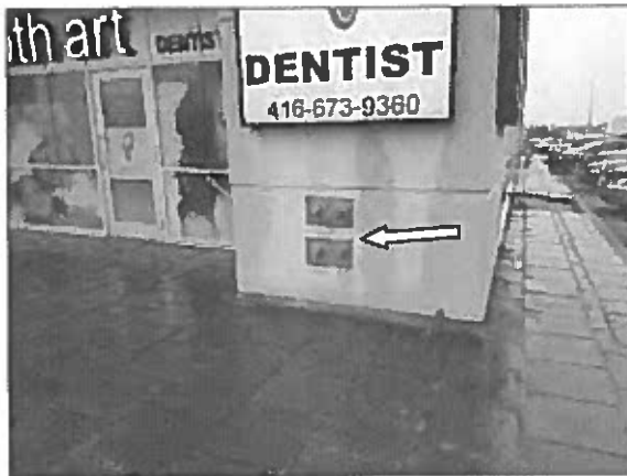
View of the fire department Siamese connections located on the south elevation of the Site Building.
