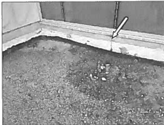
View of the damaged insulation boards and unfastened drainage boards noted on the north elevation of the Site Building.
