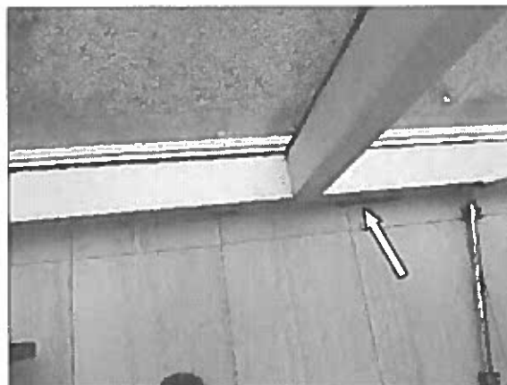
View of the cracked/missing tile grout noted in the ground floor level pharmacy.
