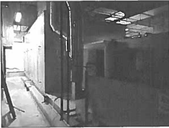
View of the "Engineered Air" MUA unit.
