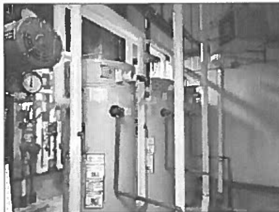
View of the "Bradford White Corporation" natural gas-fired DHW heaters.
