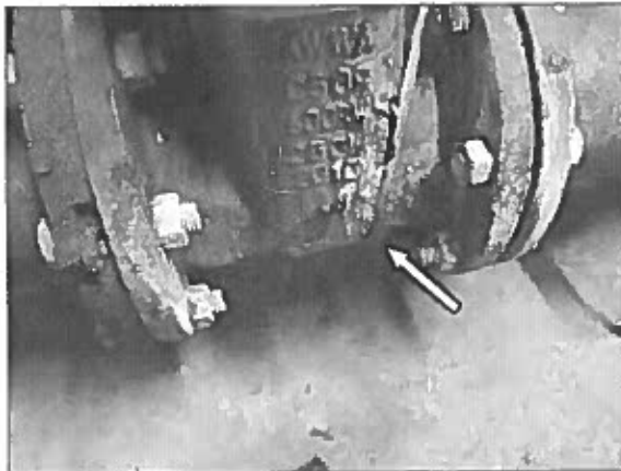
View of the corrosion on the sprinkler main piping noted within the main sprinkler room.
