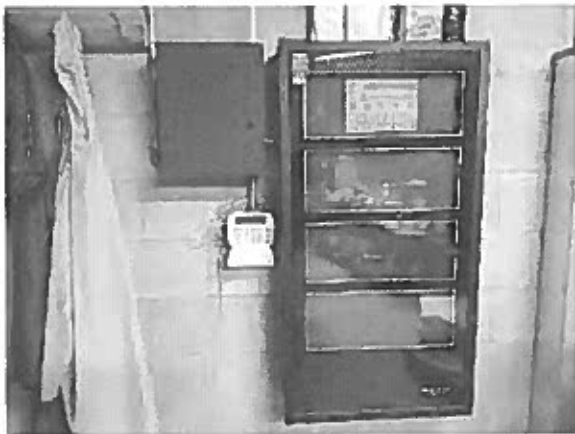
View of the "Notifier" fire alarm main control panel.
