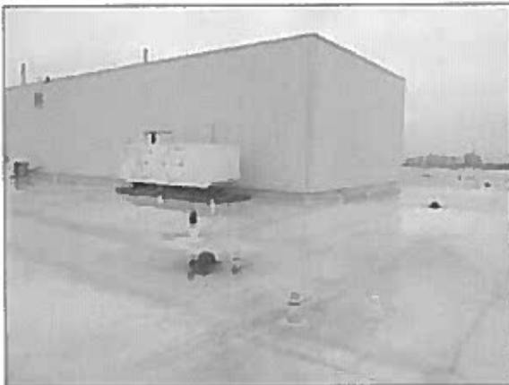
General view of the PVC single-ply membrane roof system noted on the main roof area.
