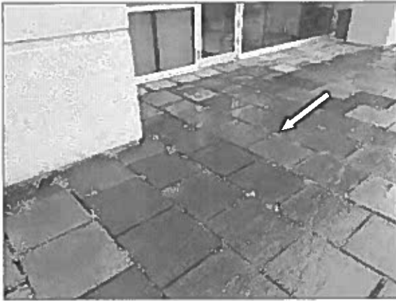
View of the vegetation growth in the interlocking stone pavers noted adjacent to the south elevation of the Site Building.
