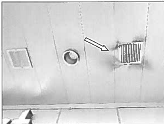
View of the staining on the metal ceiling panels noted in the main lobby of the Site Building.
