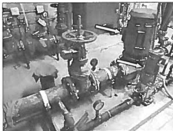
View of the "Plad" centrifugal fire pump and "Wilo" jockey pump.
