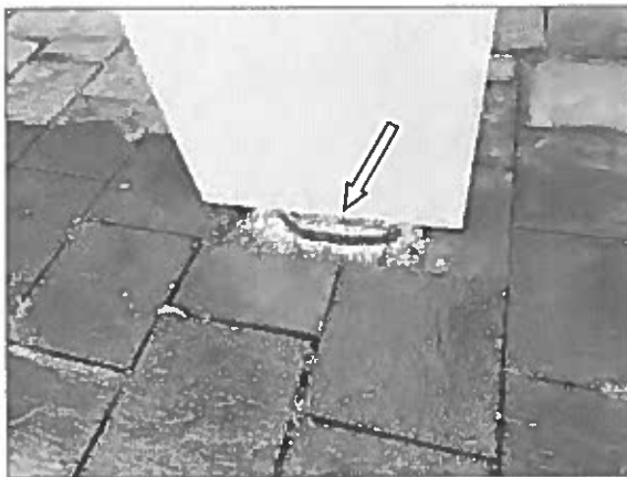
View of the exposed steel reinforcing bars in the concrete column noted adjacent to the south elevation of the Site Building.
