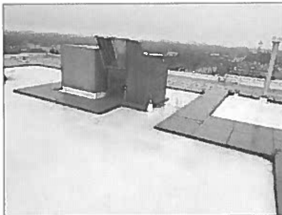
General view of the PVC single-ply membrane roof system noted on the upper roof area.
