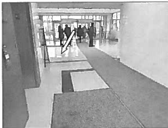
View of an anomaly in the concrete floor slab noted in the main entrance lobby.
