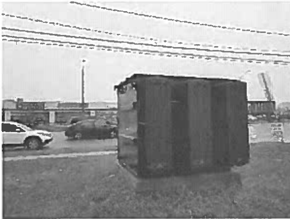
View of the concrete pad-mounted municipal transformer located on the southwest portion of the Site.
