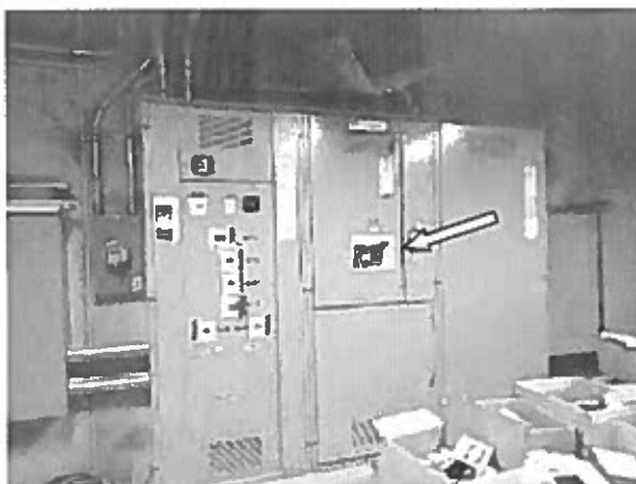
View of the “Eaton” main electrical switchgear and disconnect switch.
