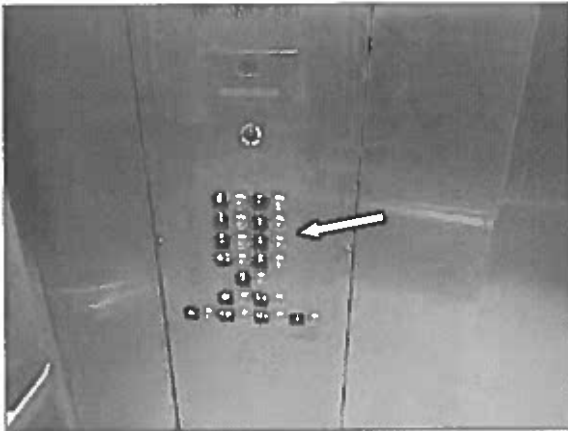
View of a typical elevator control panel within the elevator cab.
