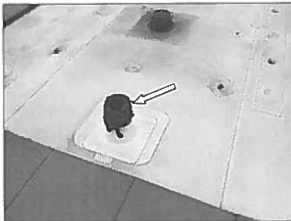
View of the plastic cover on the roof vent noted on the upper roof area.
