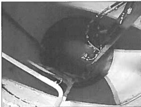
View of the in-ground concrete sump pit complete with a pump system.
