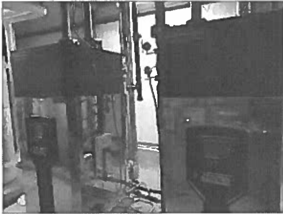
View of the “Camus DynaForce Series” natural gas-fired heating boilers.
